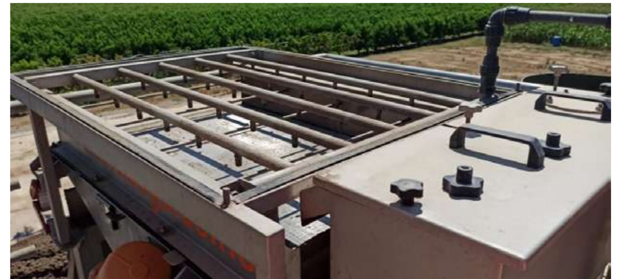
Image 3.5. Automatic cleaning tubes installed in a vibrating screen.
