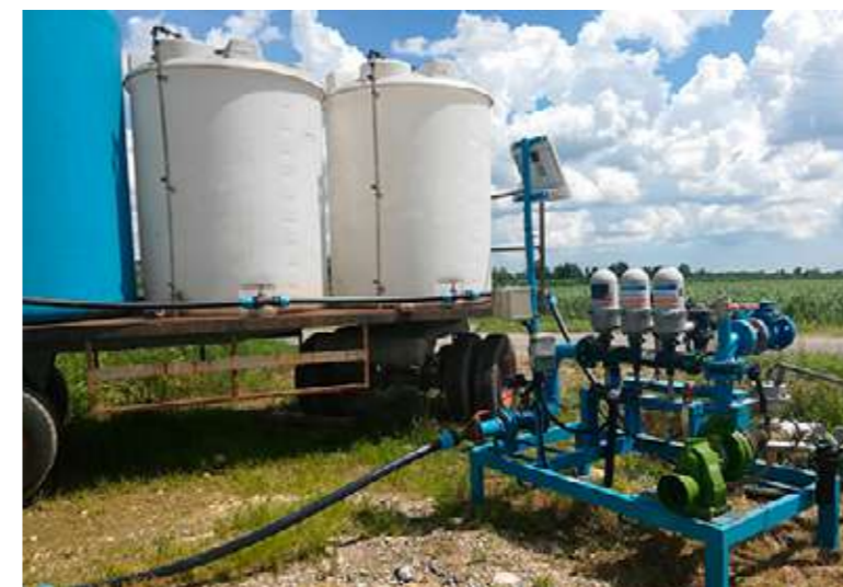
Image 6.4. The storage and pumping station for the Drip 1 transference field in Lombardy (Italy).
